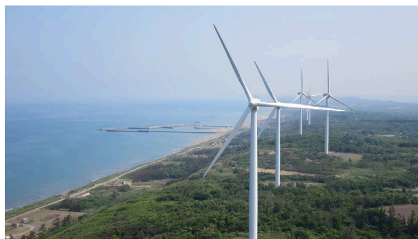
Oga is an ideal site for wind power generation, with average annual wind velocity exceeding 6 m/s at many points. (Oga wind power plant)
